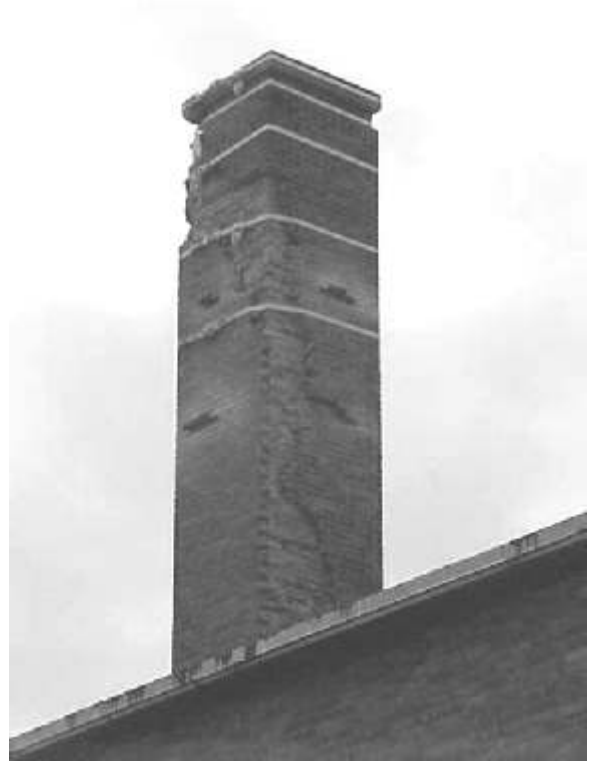
Chimney damaged by lightning
